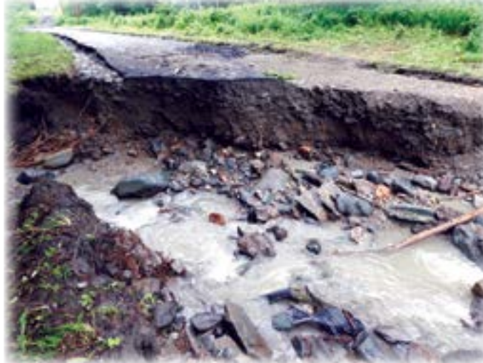
A Vermont road is washed away due to the extreme flooding experienced this summer. (Greg Whitchurch)
