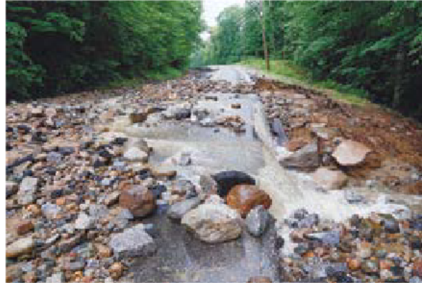
Heavy rains in July 2023 caused flooding throughout New England. Route 113 in Madison, NH was damaged with thousands of yards of gravel washed across the road making it impassable. (Rachel Sharples/Conway Daily Sun)
