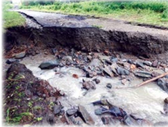
A Vermont road is washed away due to the extreme flooding experienced this summer. (Greg Whitchurch)
